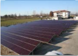
Ground mounted PV system
