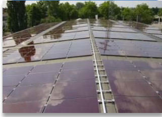
Commercial Rooftop PV system
