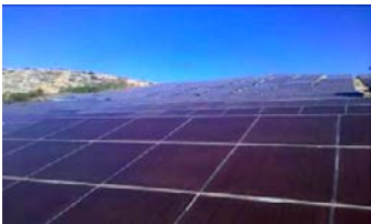
Capacity: 1MW Type: Ground Mounted Location: Yunnan, China
